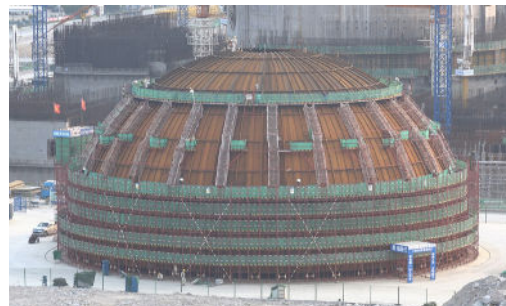
Fuqing Nuclear Power Plant, Fujian Province (2017)
